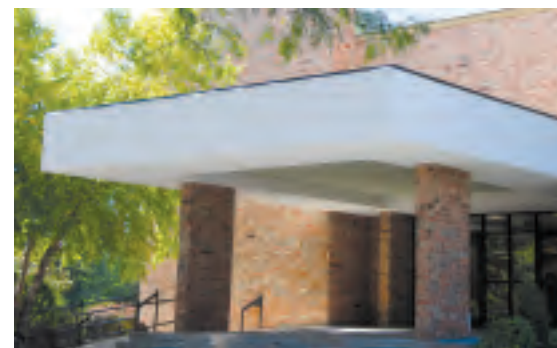
Repairs to the portico are completed. Thanks to everyone involved in this project!
